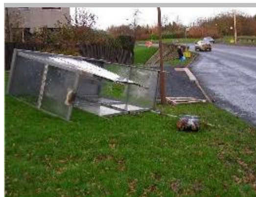
Vandalised bus stop
